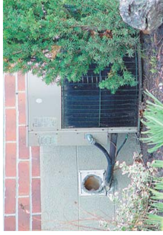
This image shows the air conditioning condenser.
